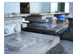
Corroded Steel Bearing
